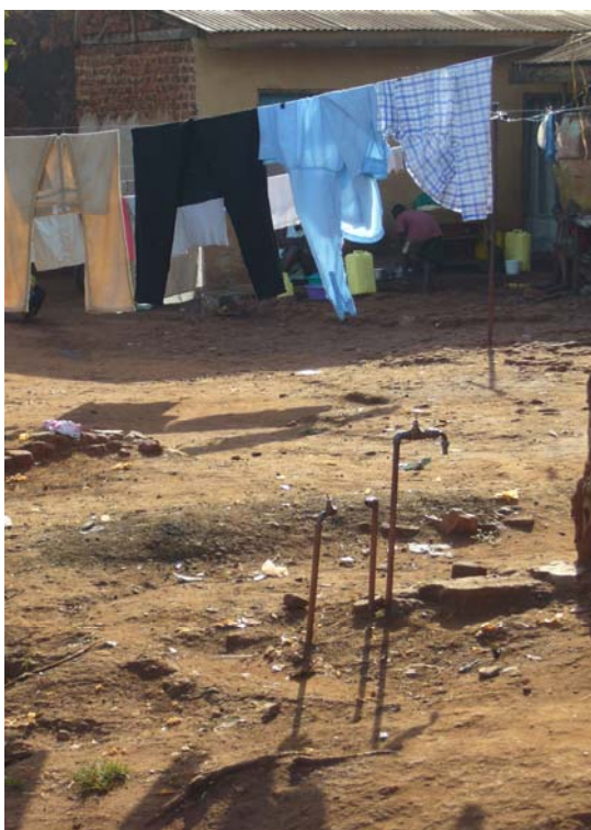
Public standpipe disconnected
