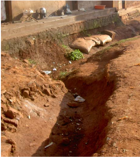
This used to be a road...
