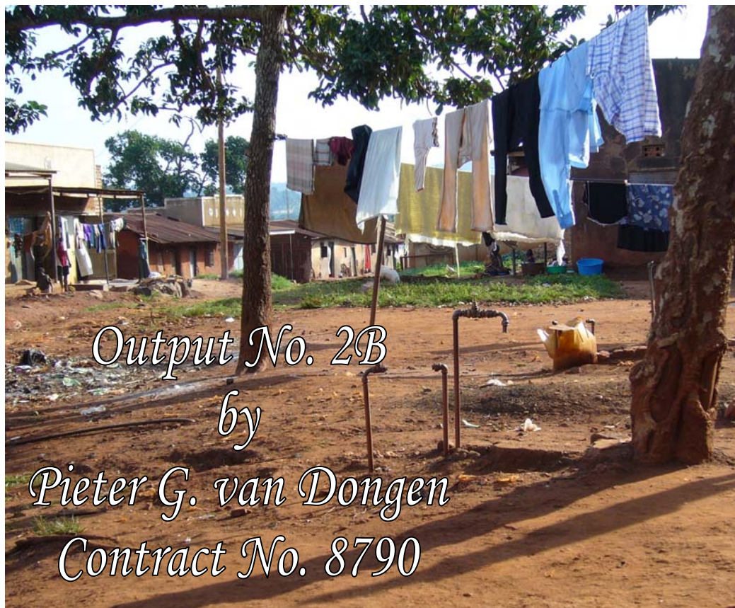
Disconnected Public Standpipe in Budumbuli West
